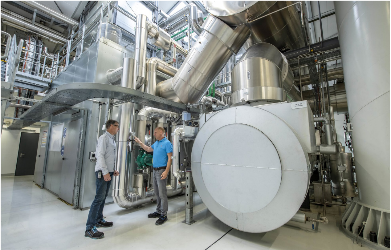
In addition to electricity, the CHP systems also produce heat, which is used during the production process or as heating. tesa will have at least four of these systems in operation by the end of 2020.
